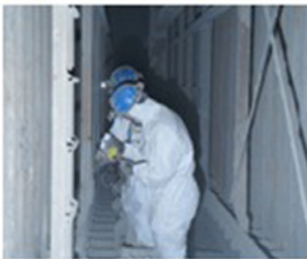
ESP Services PLTU 2 BANTEN LABUAN (2X315 MW) PLTU PALABUHAN RATU (3X350 MW) PLTU JERANJIANG (3X25 MW) PLTU TENAYAN (2X110 MW) PLTU TANJUNG JATI B UNIT 1 & 2 (2X660 MW), etc
