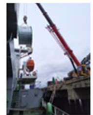
Instalasi Belt Conveyor PLTU TANJUNG AWAR-AWAR (2X350 MW) PLTU PAITON 9 (1x660 MW) PLTU BANJARSARI (2x135 MW) BAHTERA ADIGUNA
