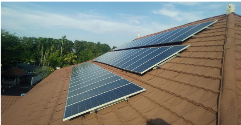
▶▶ ROOFTOP SOLAR PV - PLTS Bali
