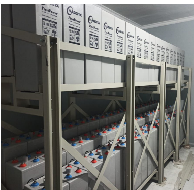
▶▶ BATTERY BANK - PLTS Messah
